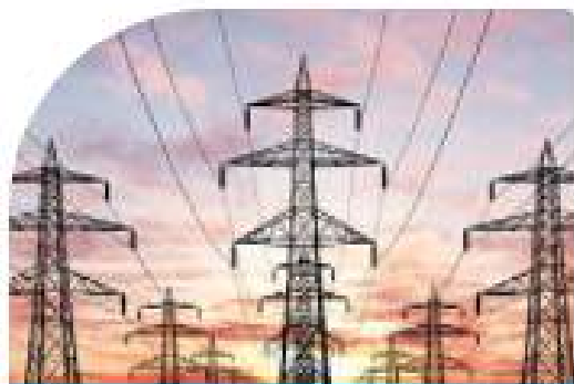
07. Transmission and Distribution
